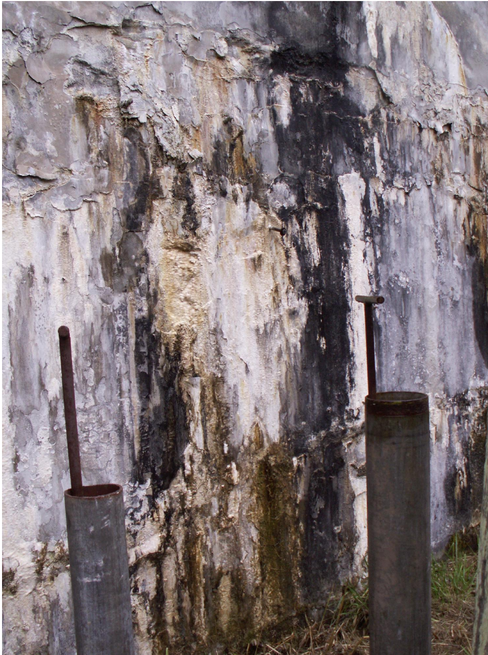
Photo No. 19 View of typical delaminating of patch concrete on downstream side of dam
