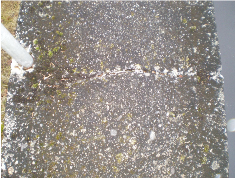
Photo No. 7 View of crack 2 on crest of dam
