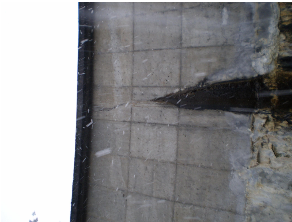
Photo No. 14 View of crack 5 on downstream side of dam
