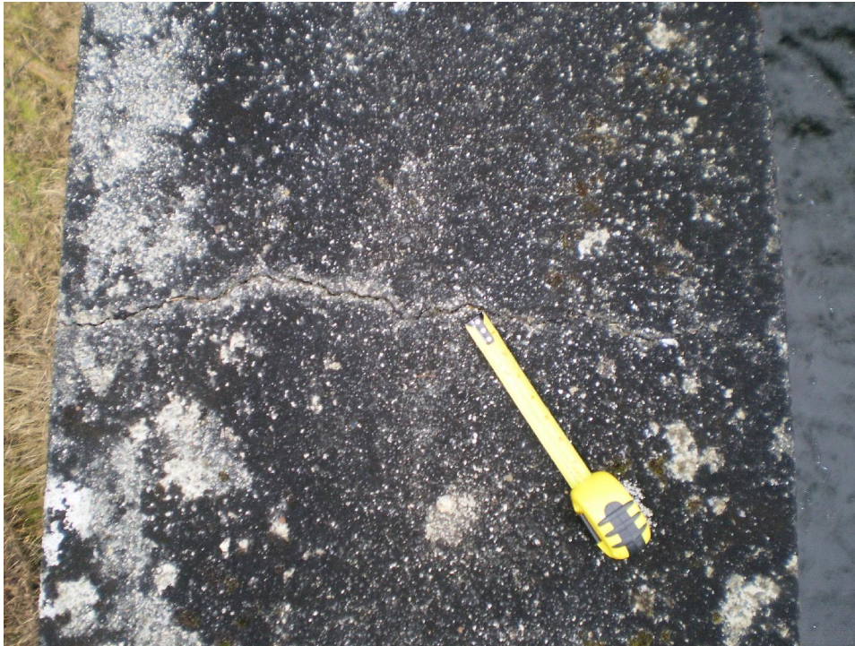
Photo No. 13 View of crack 5 on crest of dam
