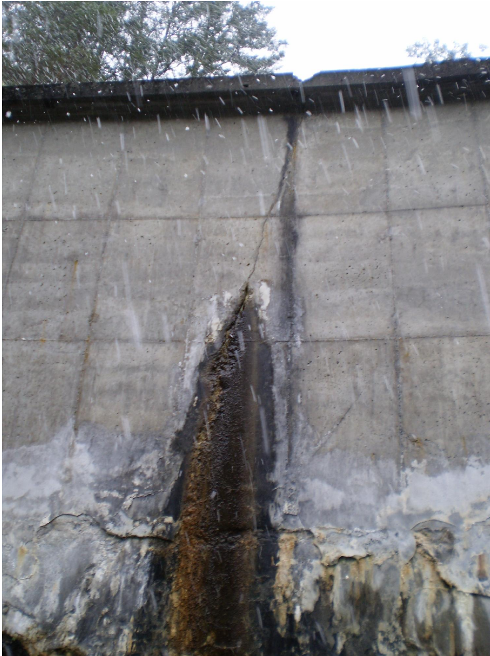
Photo No. 18 View of crack 7 on downstream side of dam
