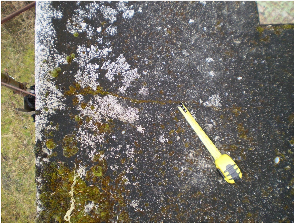
Photo No. 11 View of crack 4 on crest of dam
