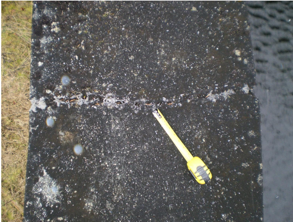
Photo No. 15 View of crack 6 on crest of dam
