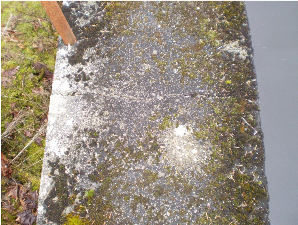
Photo No. 5 View of crack 1 on crest of dam
