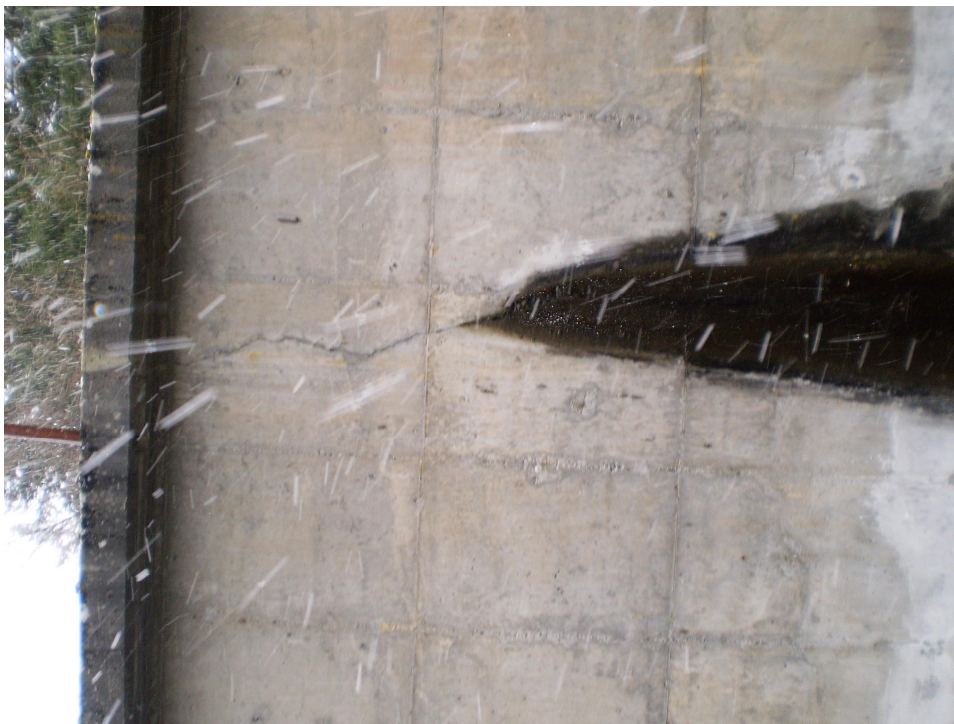
Photo No. 6 View of crack 1 on downstream side of dam
