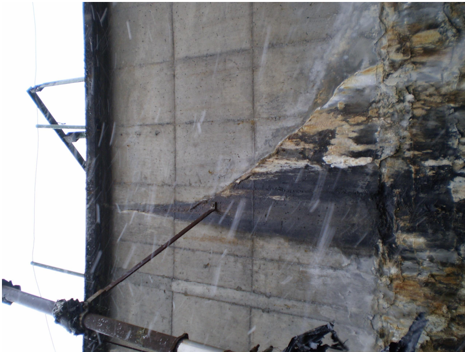
Photo No. 12 View of crack 4 on downstream side of dam
