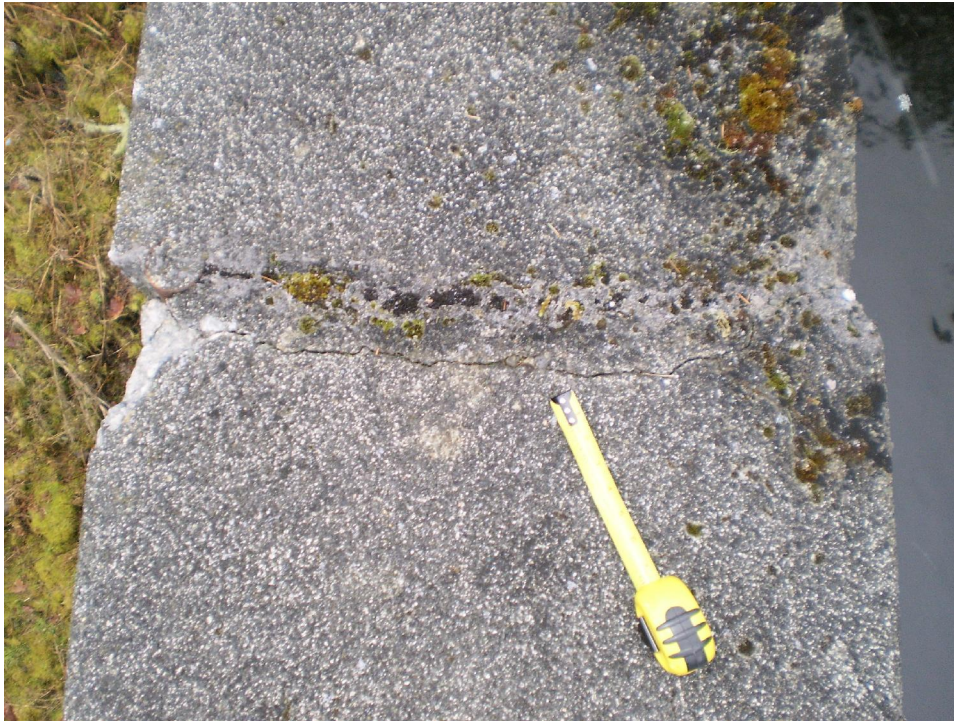
Photo No. 17 View of crack 7 on crest of dam
