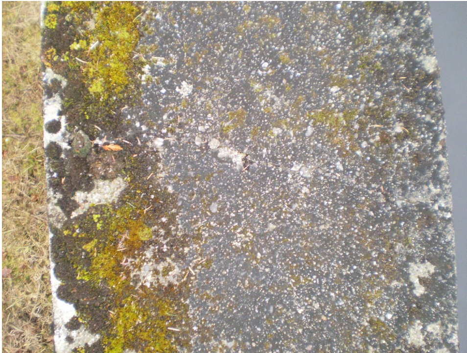
Photo No. 9 View of crack 3 on crest of dam
