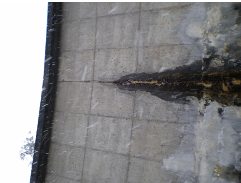
Photo No. 16 View of crack 6 on downstream side of dam
