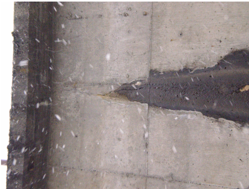
Photo No. 10 View of crack 3 on downstream side of dam
