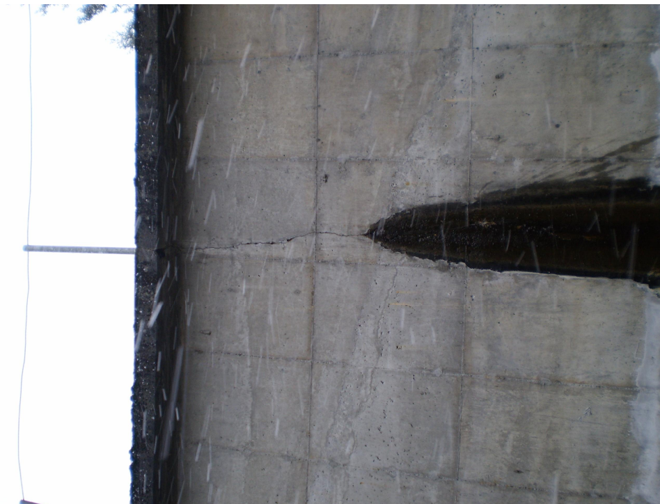
Photo No. 8 View of crack 2 on downstream side of dam
